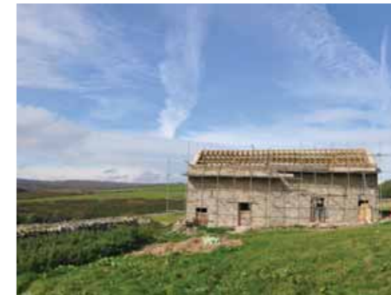
Holgate Moor barn, near Barningham, a dramatic landscape feature with a roofing problem
