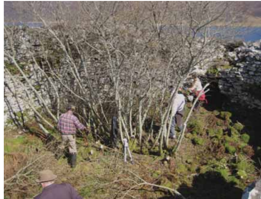
Local volunteers clearing scrub from Carroll Broch Sutherland. Under current funding arrangements Historic Scotland supports work on an average of 14 scheduled monuments and 8 smaller projects a year. © Crown Copyright, reproduced courtesy of Historic Scotland
