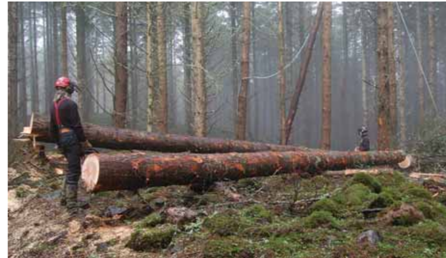
The felled trees are lowered to the ground and cut in two, supported on log 'bearers' for support and to prevent damage to the masonry. These long saw logs are left in situ for removal by Harvester
