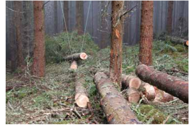
The remaining crown of the tree is then processed in the cradle and removed
