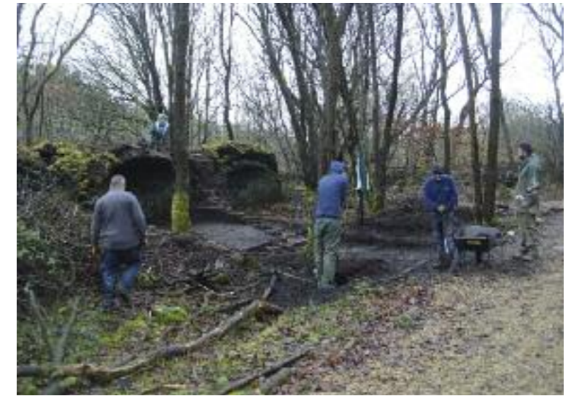
Volunteers at work near the upstanding coke oven remains © Archaeological Research Services Ltd
