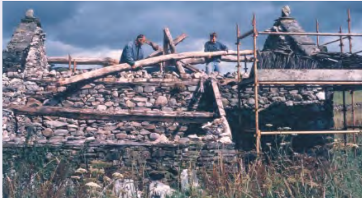
Repair work provides local employment and keeps craft skills alive. Ecclerigg Barn under repair. © Andy Lowe, Lake District National Park
