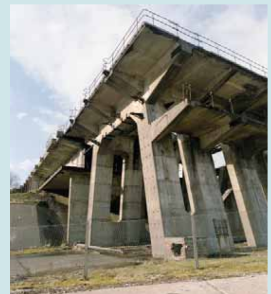
RAF Spadeadam, Cumbria, Greymare Hill. The remains of the Blue Streak missile stands are some of the country's most imposing Cold War monuments. Crown copyright. NMR
