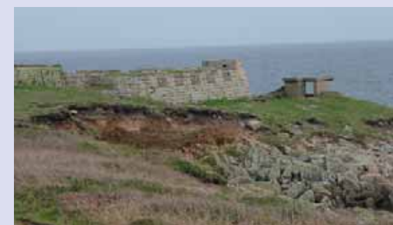
The threat from coastal erosion at The Garrison, St Mary's Isles of Scilly
