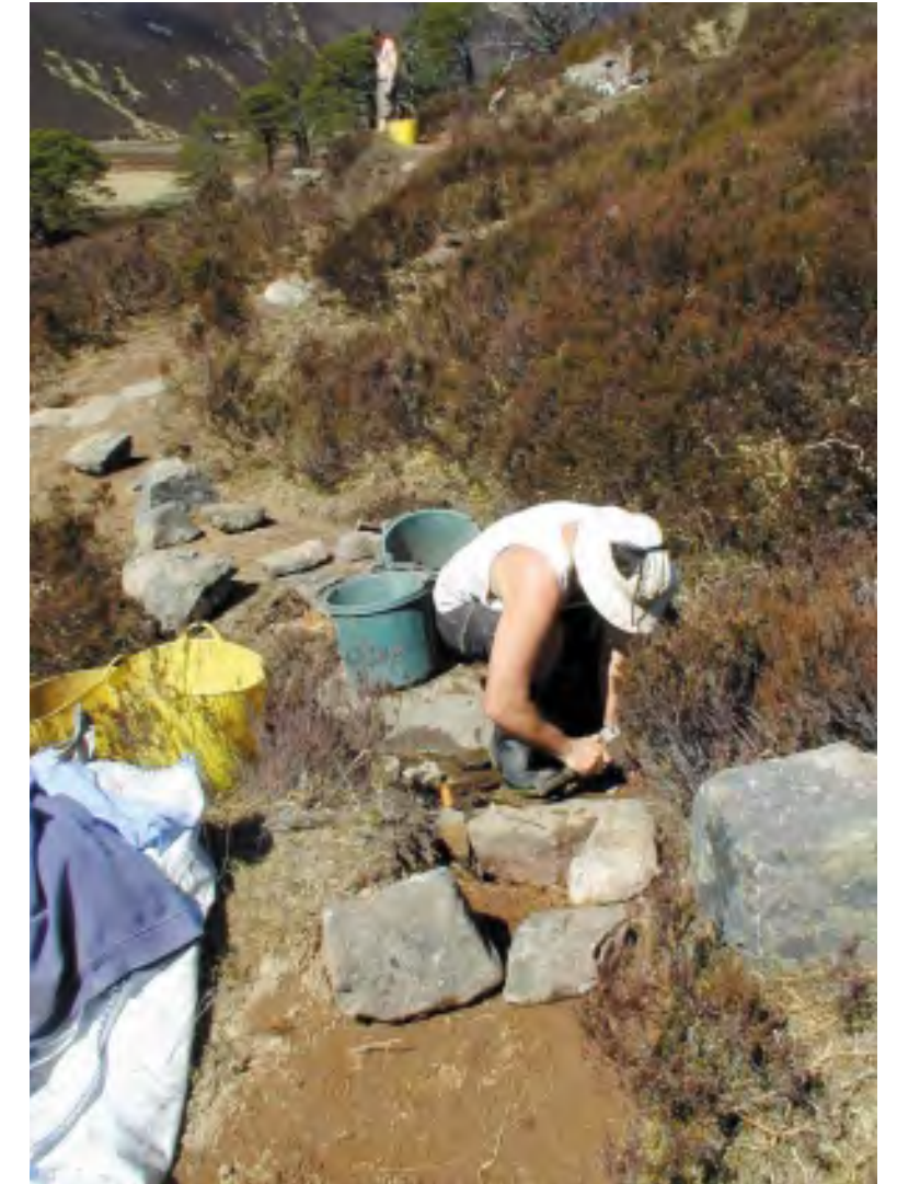
Footpath works undertaken by the NTS: the lithic scatter, sealed under peat, was discovered during this type of operation. (Photograph: NTS)
