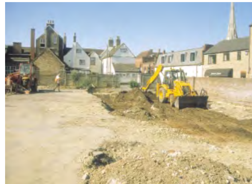
Excavations in St Ives, Cambs, were so close to the boundary of a pub that the Party Wall Act was invoked and agreement had to be reached on how close excavations could come to the wall. © Northamptonshire Archaeology
