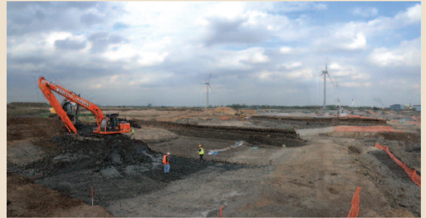
Large scale excavation of the channel deposits employing the long-arm machine method © CAU
