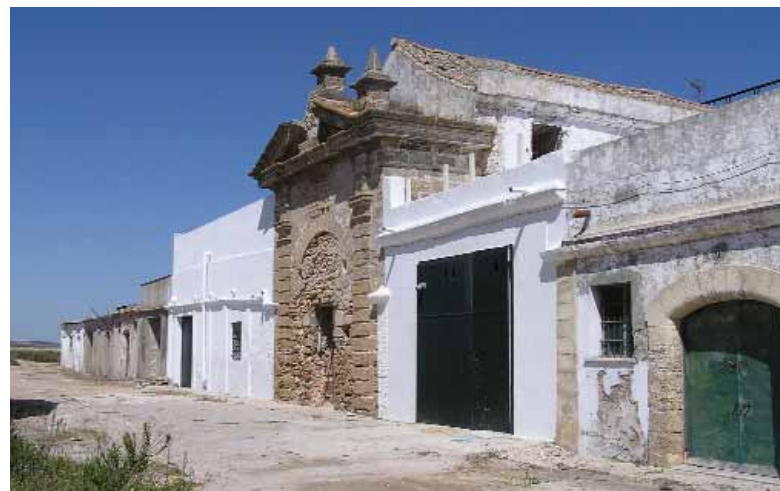
Detail of the central feature of the Real Carenero façade, Cadiz. © English Heritage
