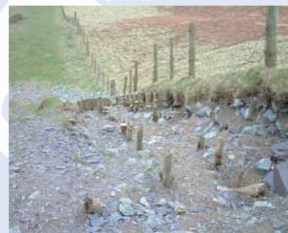
North side erosion with remains of previous (unsuccessful) repair work
