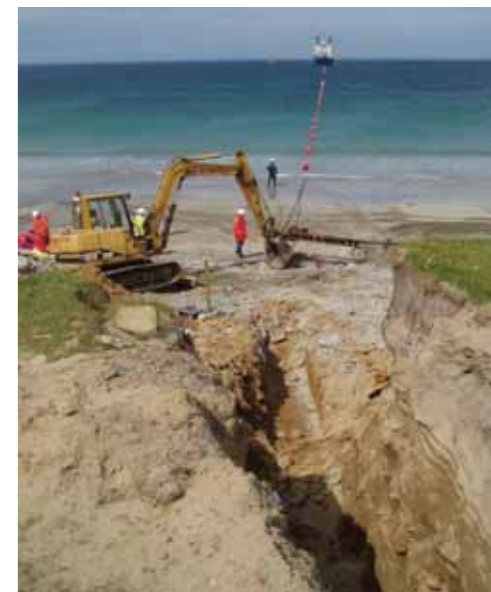
ORCA monitoring cable landfall at Skaill Bay, Orkney © ORCA
