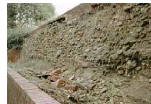
The city wall at Cecil Street is in poor condition due to severe erosion and collapse. (Photo: City of Lincoln Council)
