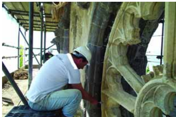
Mason at work on the Bathstone wheel window. Spokes damaged beyond repair have been removed ready for insertion of replacements (as in the right of the picture). After cleaning, the window was given a 'shelter coat' of lime to act as a sacrificial surface to protect the original stonework
