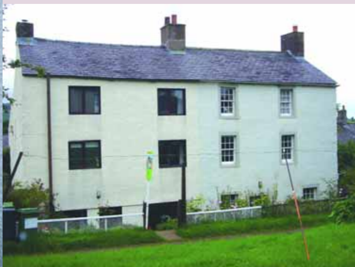
The Bad: instructive comparisons between the two halves of the same 19th-century Lake District dwellings. One way to measure which conservation areas are under threat is to look at properties whose character has been eroded by alterations to window openings and replacement of traditional windows
