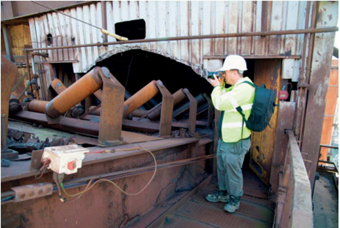
Blast furnace charging conveyor ©TEP
