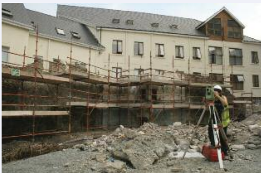
Urban excavation and survey of Waterford City Walls (Rubicon Heritage Services Ltd)
