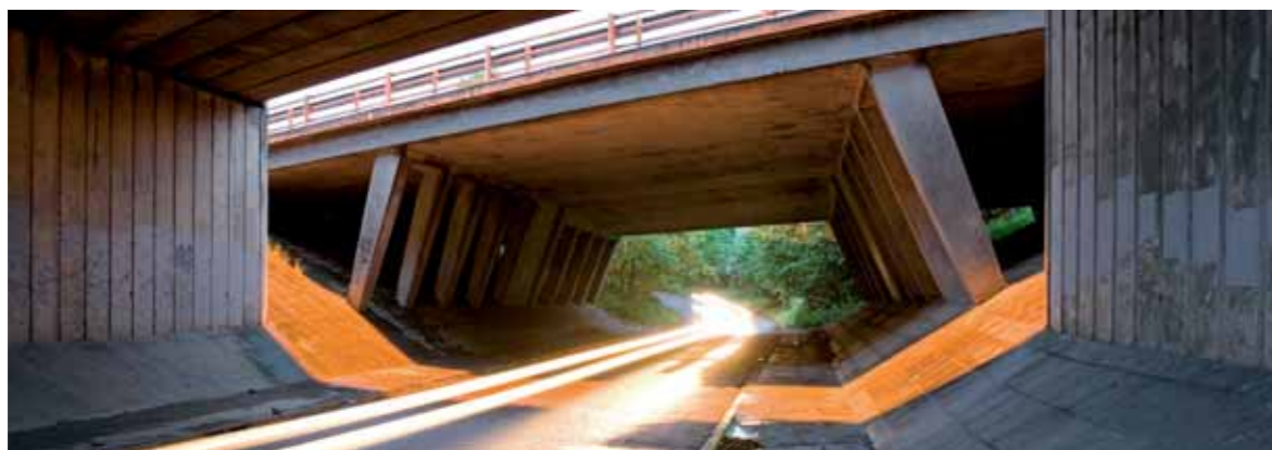
The Nicky Line Underbridge of the M1 in Herts. Photograph: Matthew Walter
