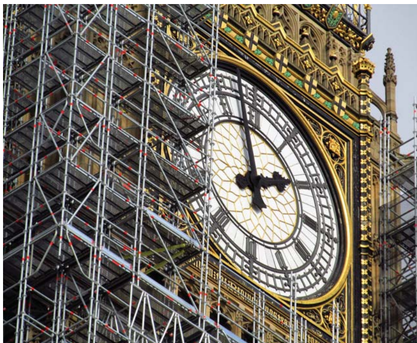
As the sector lobbies to influence big changes to archaeology inside the Palace of Westminster, so do we to ensure that repairs to the exterior of the historic seat of Parliament include archaeological investigation. Credit: London October 20 2017 (53) Scaffolding Big Ben by DAVID HOLT is licensed under CC BY 2.0 ( https://flic.kr/p/ZBQY5V )
