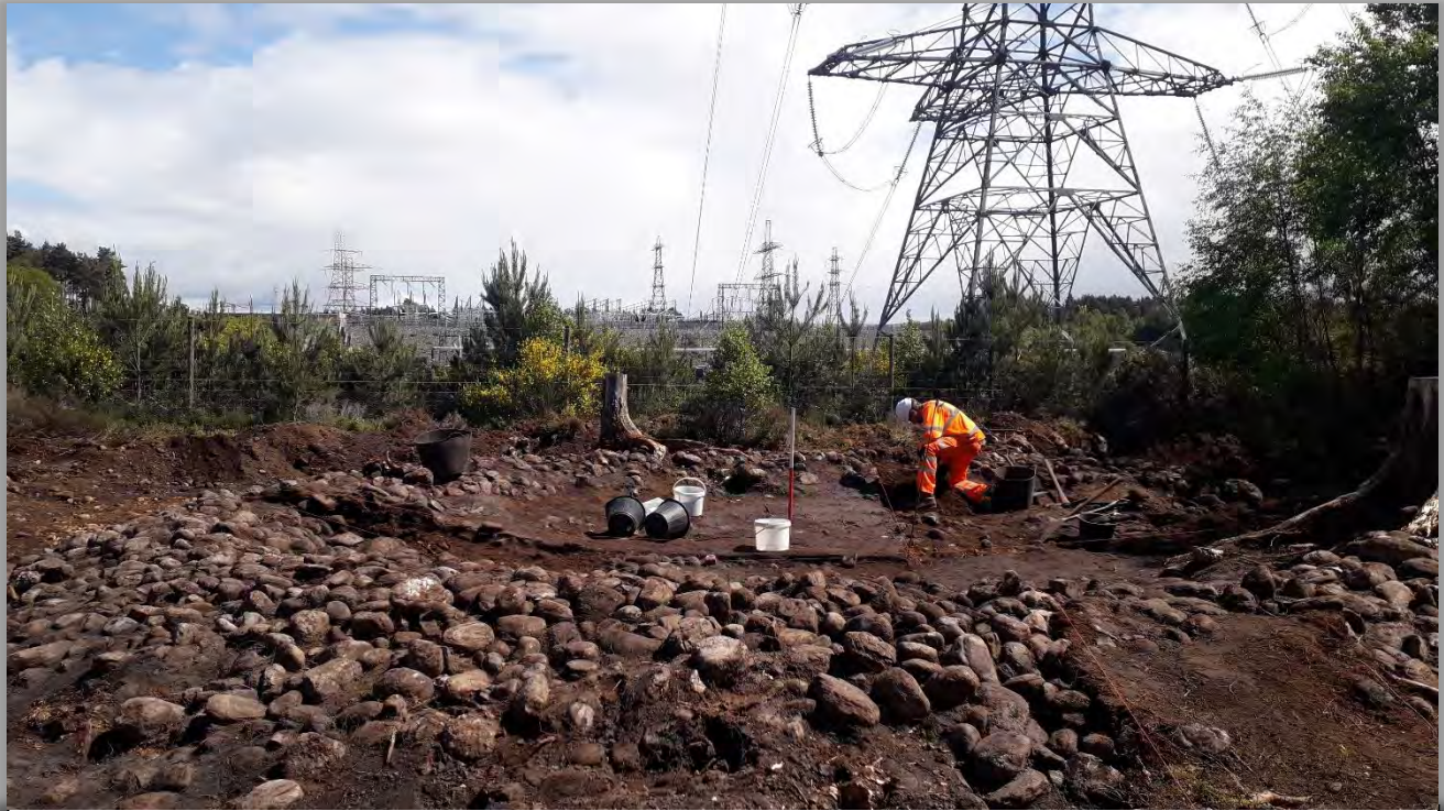
Excavations were part of a site survey for a new extension to the existing Beaully substation
