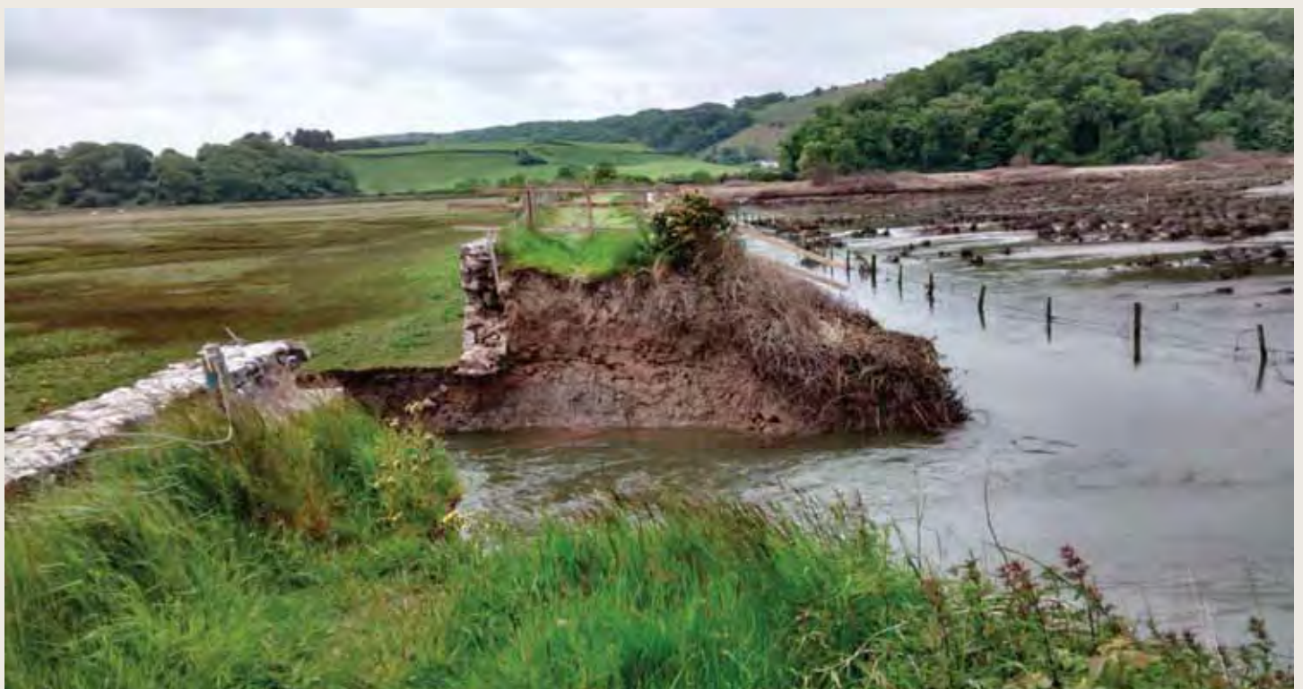
Photograph showing the breach in the bank and where the phases of construction can be seen. Credit: Judith Doyle
