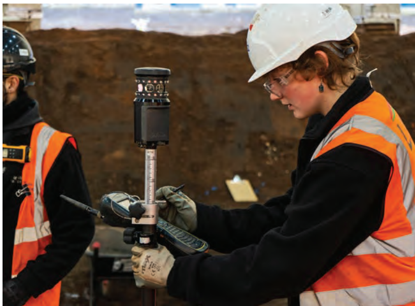
Trainee Eleanor surveying – Trainee programme 2018 LM/MHI with the West Midlands Combined Authority and BMet. Credit: LMJV
