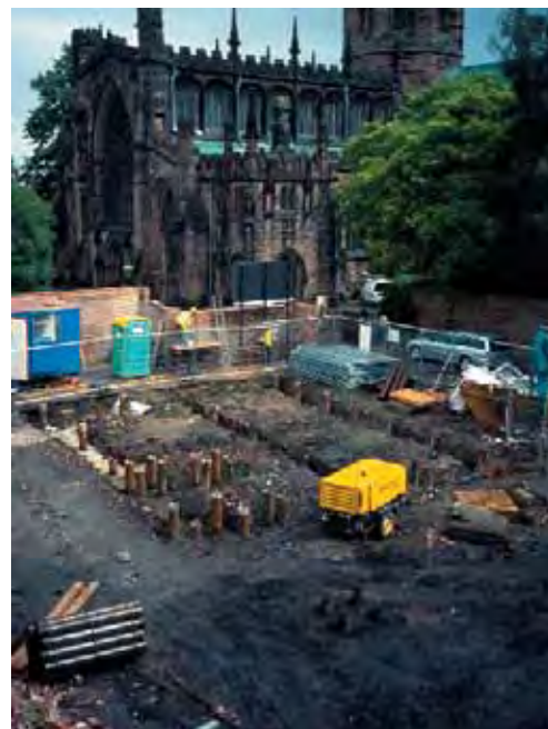
Excavations at the Lamb Hotel with remains of Anglo-Norman timber structures, and piling in progress © Gifford
