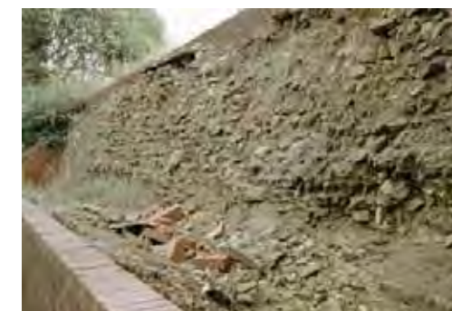
The city wall at Cecil Street is in poor condition due to severe erosion and collapse. (Photo: City of Lincoln Council)
