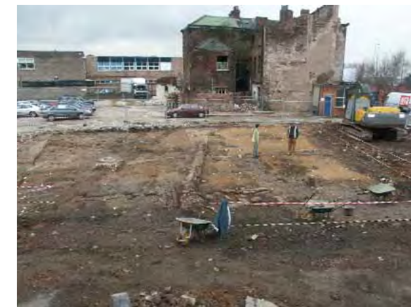
Part of the Abito development site, excavated by the University of Manchester Archaeological Unit in 2005. Remains ranged from 13th-century rubbish pits and property boundaries to industrial period back-to-back and blind back workers' housing
