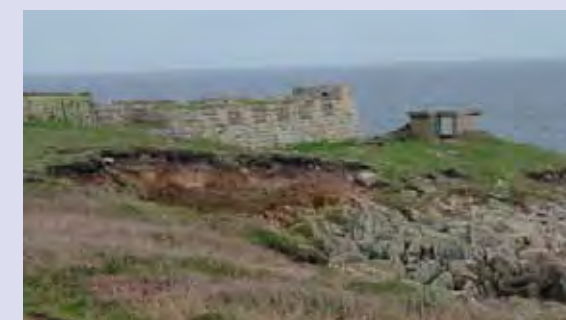
The threat from coastal erosion at The Garrison, St Mary's Isles of Scilly
