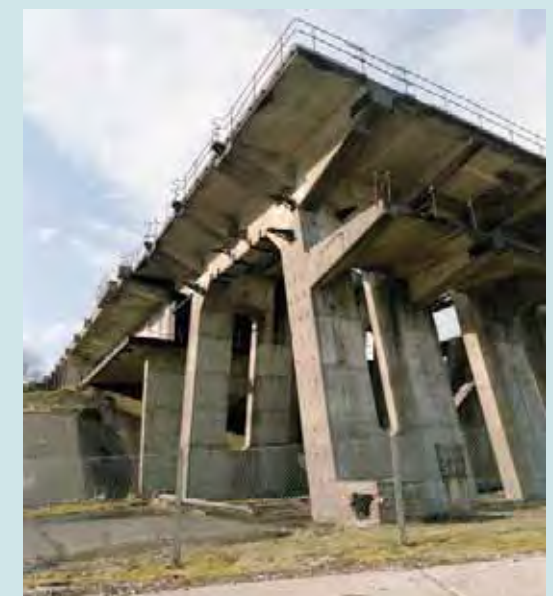
RAF Spadeadam, Cumbria, Greymare Hill. The remains of the Blue Streak missile stands are some of the country's most imposing Cold War monuments. Crown copyright. NMR
