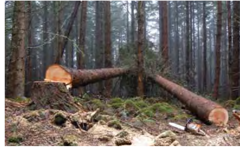
Trees now supported safely over dun wall and at a good working height for processing
