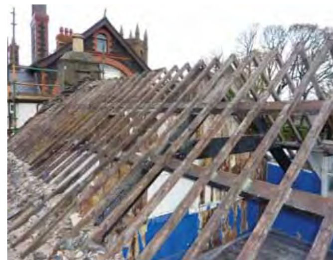
Rehanging the original slates on this early 19th-century cottage in Kirk Michael revealed a carefully made roof whose precision carpentry belies its low status. Note the vertically boarded timber partitions in the upstairs rooms
