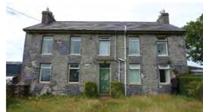
Ballavagher, a Manx farm probably improved in the second quarter of the 19th century on the back of rising demand for dairy products in the nearby capital, Douglas. Spoiled by modern windows and loss of interior detail, its slate-hung façade is a rare local example. The house is likely now to be saved within a business park development
