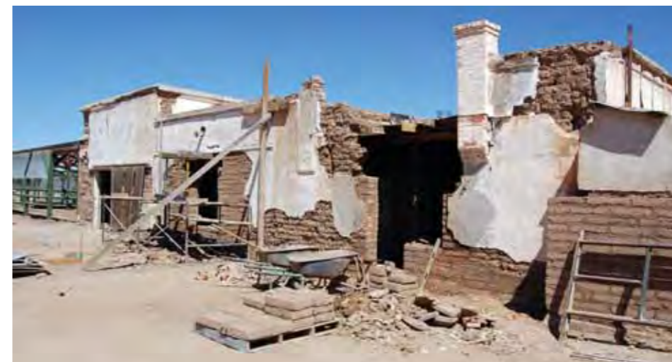
Canoa ranch buildings immediately after purchase by Pima County © Simon Herbert, Pima County
