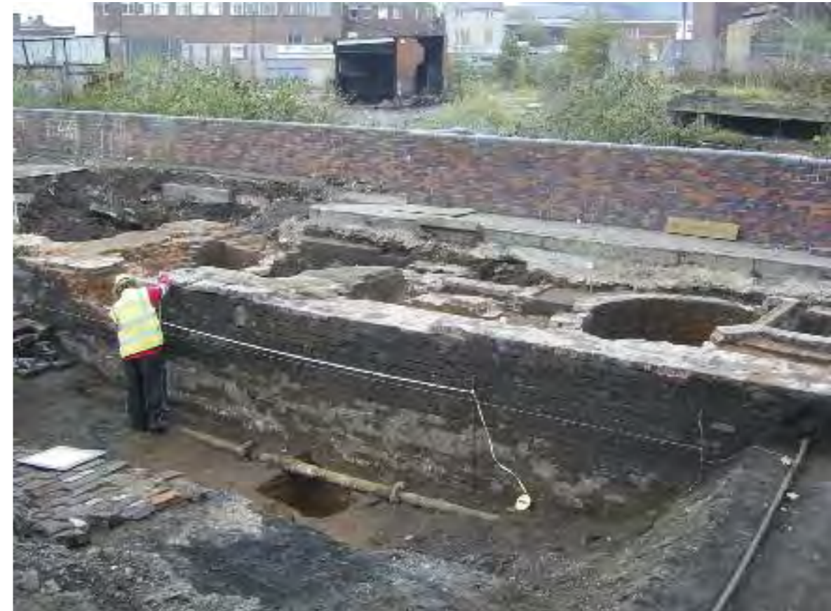
Ashted canal pumping station at Eastside Locks under excavation. © Birmingham City Council
