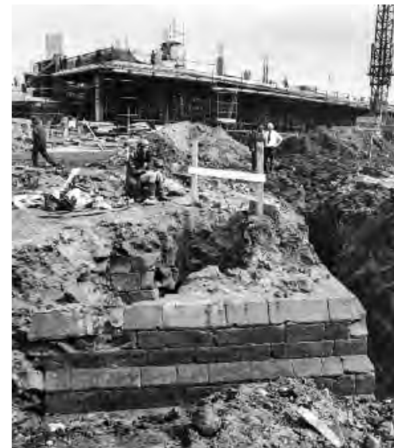
Stone wall exposed during construction of the Wholesale Markets on the manor house site. © Birmingham City Council
