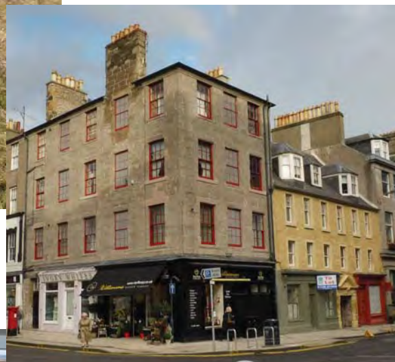
(above) Late 17th-century and 18th-century buildings on Perth High Street following conservation repairs. Credit: PKHT
