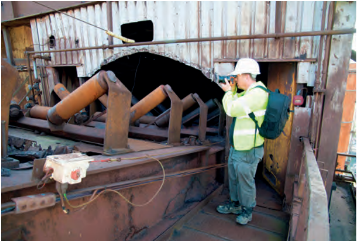
Blast furnace charging conveyor ©TEP
