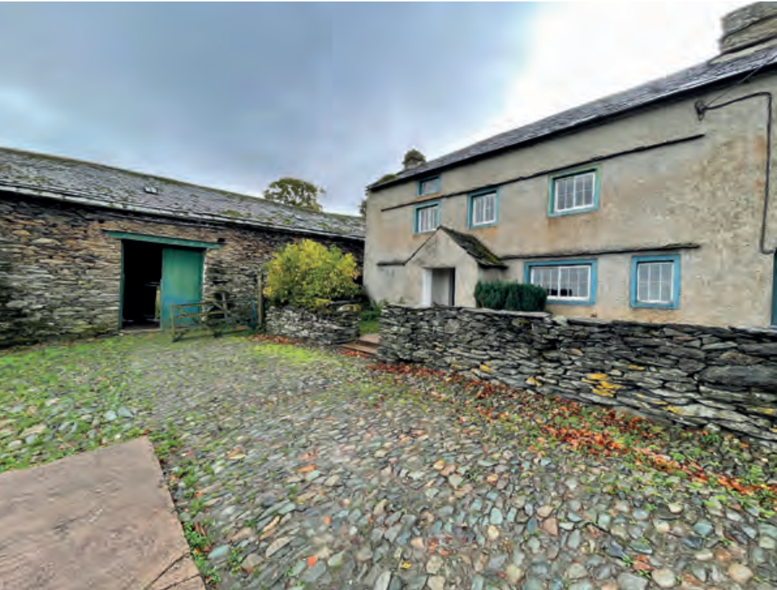
Front elevation of the farmhouse, with the south barn to the left ©www.parti.global
