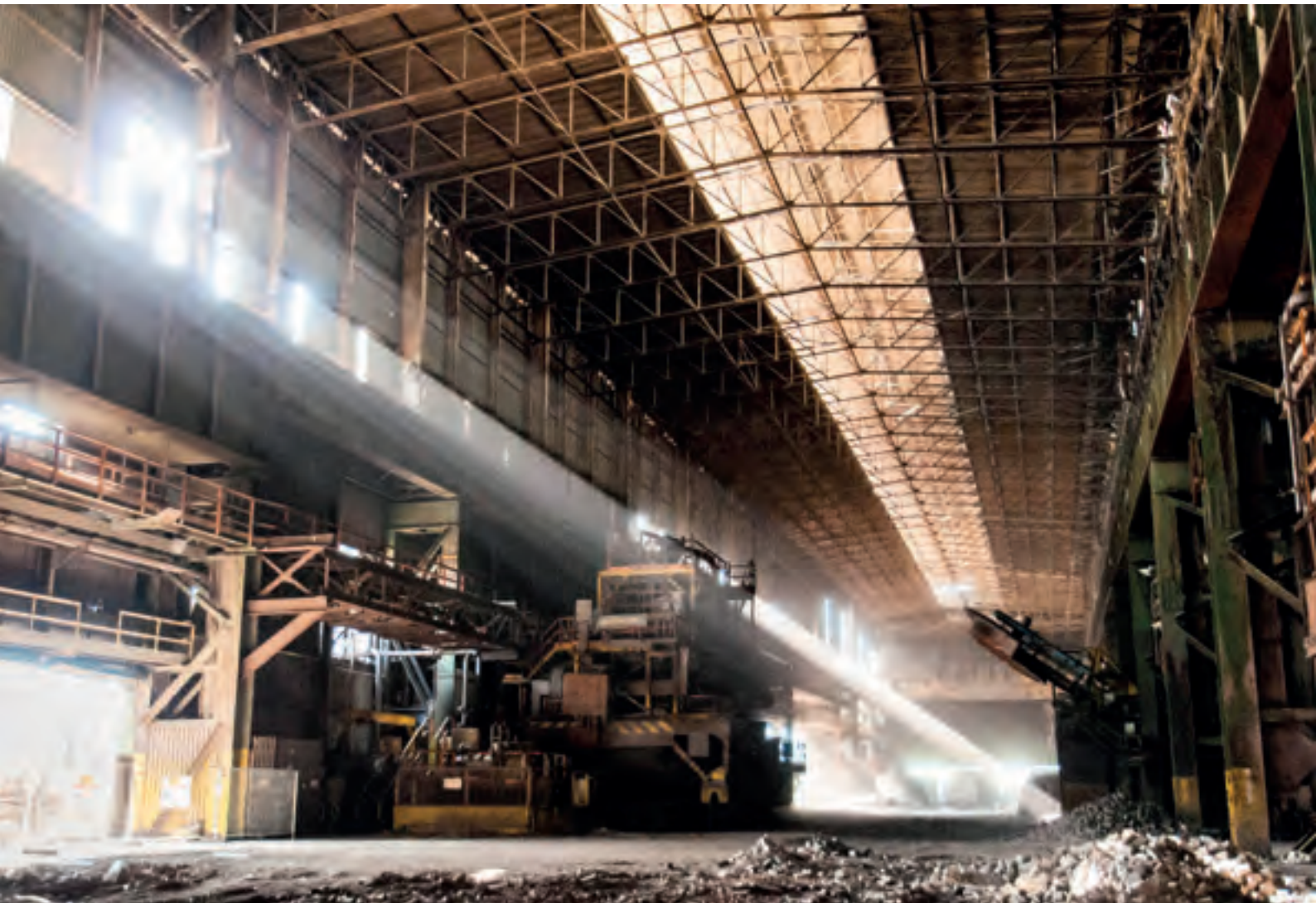
BOS Plant Teeming Bay, showing a de-gasser unit ©TEP
