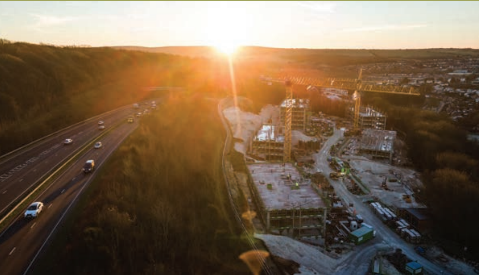
Aerial view of busy construction site in morning sunlight close to Brighton, East Sussex, UK. Credit: P Babic (Shutterstock)
