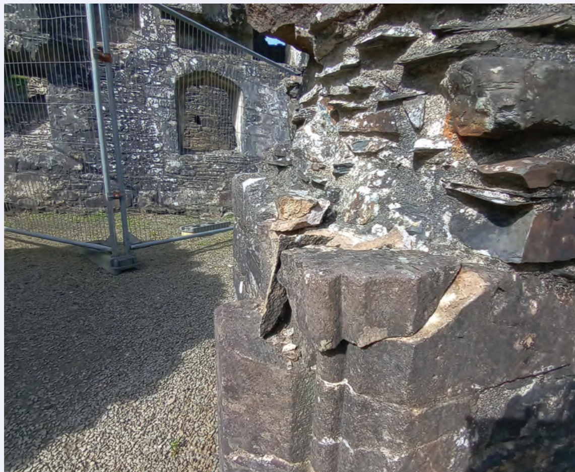
Damage to Okehampton Castle caused by antisocial behaviour, West Devon, NHLE list entry 1165647. Credit: Devon & Cornwall Police
