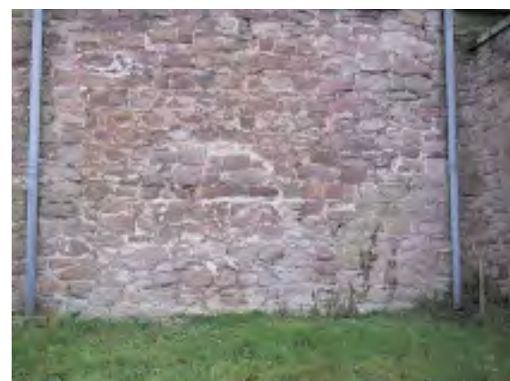
Traces of the arch of the cloister vaulting can be seen on the exterior of the north wall of the north aisle
